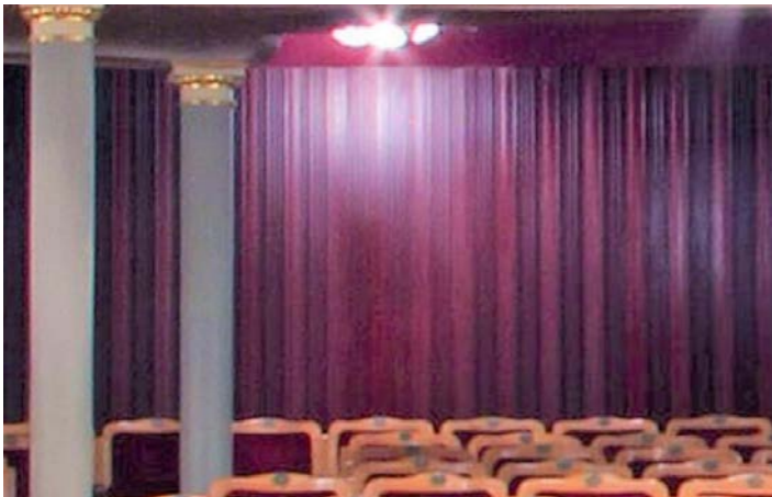
Picture 2. Installation of diffusion panels of the semicircular back wall behind the under-balcony space in the hall's stalls
